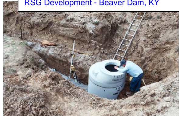
Installation of Sewer Line and Lift Station RSG Development - Beaver Dam, KY
