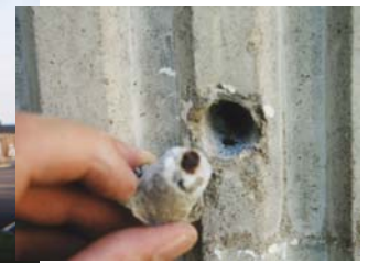
Post Tornado Structural Assessment Roosevelt House I & II, O'boro, KY Client: Monroe Guarantee Ins. Co.
